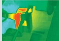
Motor: Bearing Problem
